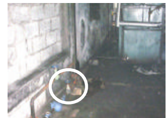
Efficient Steam Distribution ( Steam Traps)
