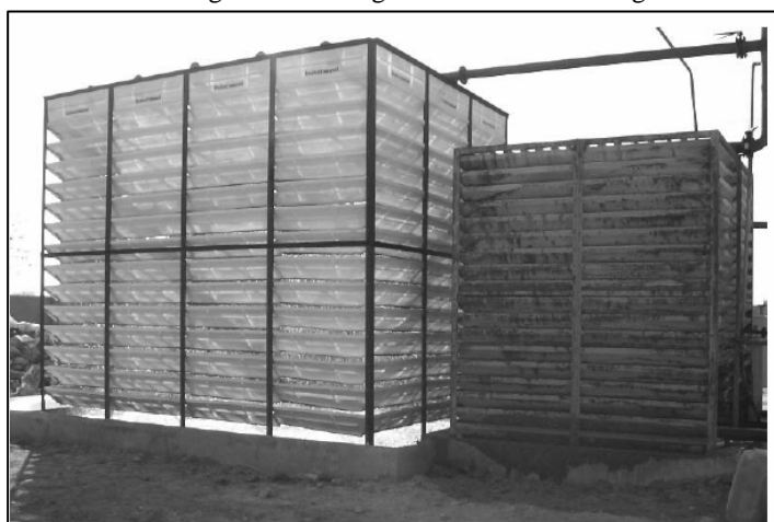
New Cooling Tower Along side The Old Cooling Tower
