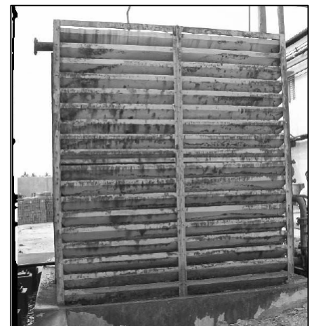
Old Cooling Tower
