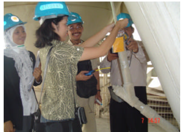
Figure 6: Marking of Leak
