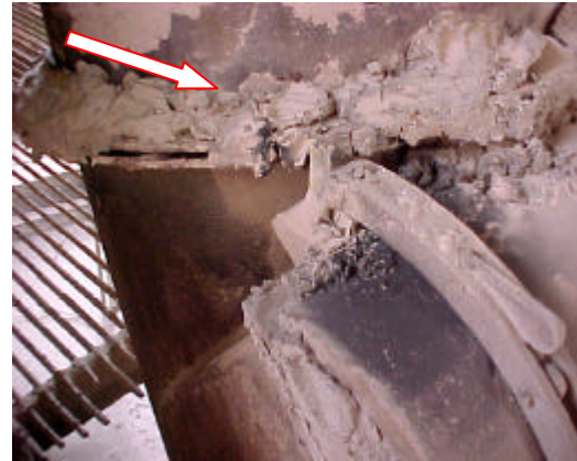
Figure 3: Leaks source at down pipe; flange is open
