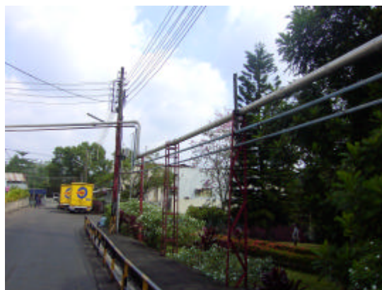
Figure 1: Insulated steam pipelines at AMW
