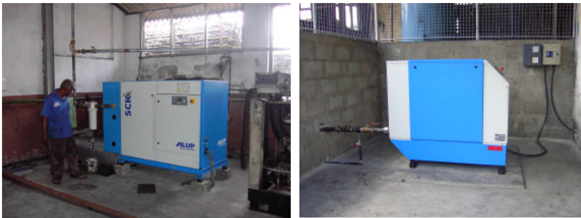
Figure 1: the New Compressors
