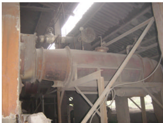
Figure 1. Stack economizer installed on coal fire boiler
