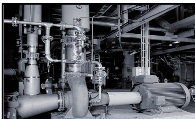
Figure 1. A Pumping System in an Industry (US DOE, 2001)
